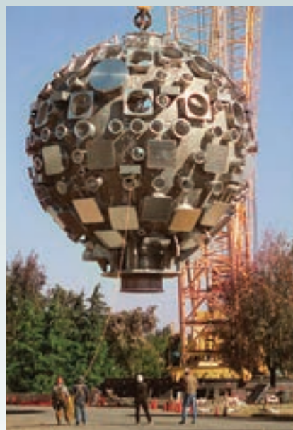
The NIF’s spherical target chamber is hoisted by crane for final placement during the facility’s construction.
