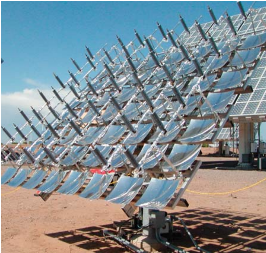
Figure 4. Concentrating Technologies 1-kW system installed at Arizona Public Service site in Phoenix, Ariz. This is the first grid-connected system using multijunction solar cells. The narrow cylinder seen in front of each mirror is a heat radiator, at the bottom of which the receiver cell is mounted.
